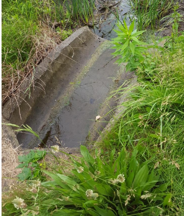
Figure 3- outfall that is conveying grass clippings into the pond from the lined concrete channel above.
