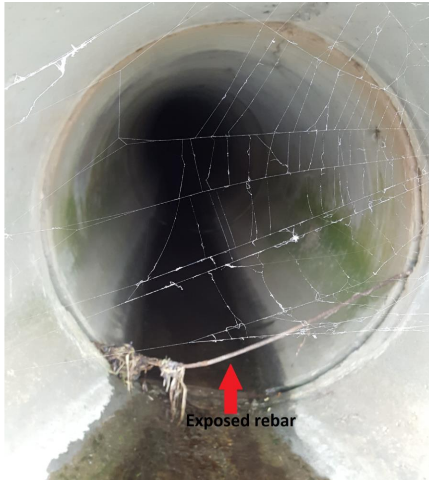
Figure 5- Rebar is exposed in the southwestern outfall that drains into the pond.
